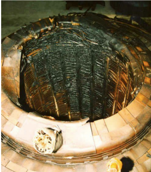
Figure 7 Evidence of increase heating within the core of a transformer winding due to harmonic currents
